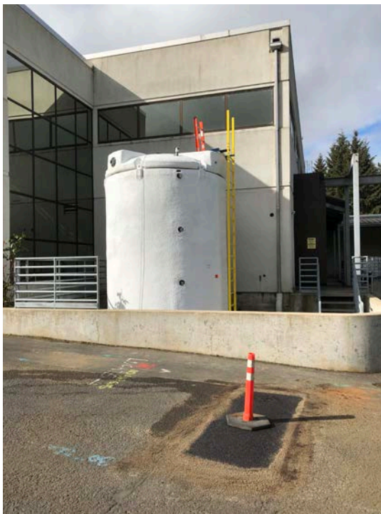
Water Treatment Plant
