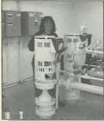
New Hawthorne pump station. Sandy Cook, Engineering Technician
